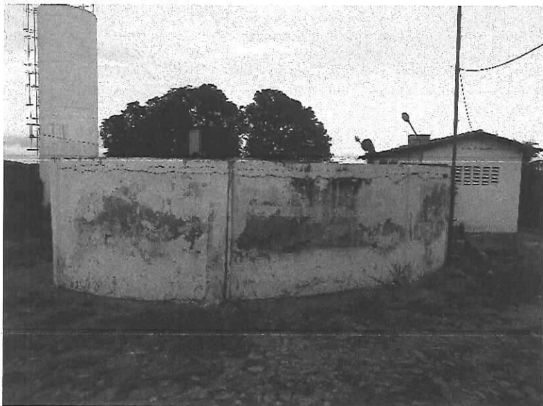
FIGURA 24 - RESERVATORIO SEMI ENTERRADO 45M 3
